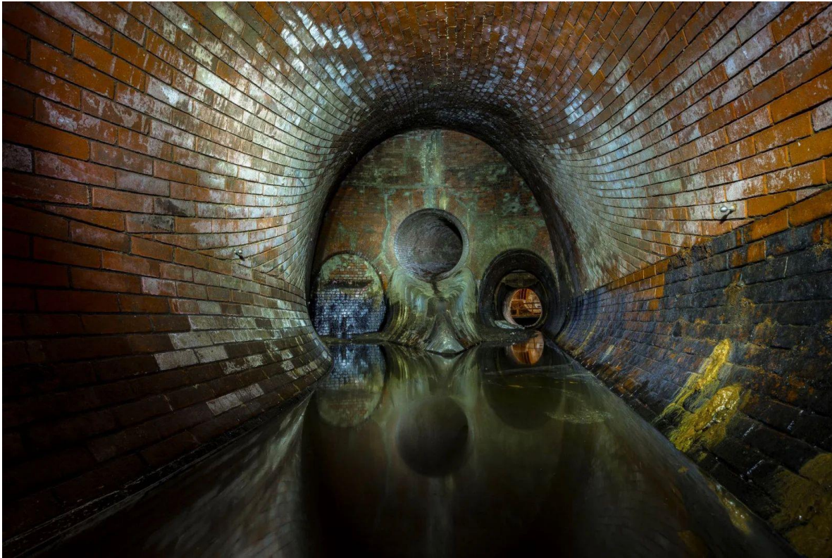
Prague sewer system – old municipal wastewater treatment plant
