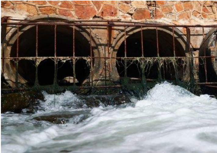
Sewage overflow during rainfall (6000 CSO in CZ)
